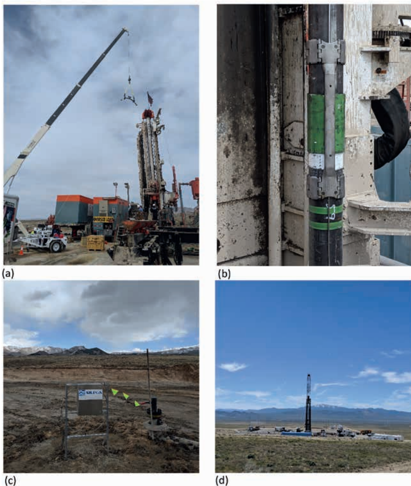
Figure 7 (a) Installation of ¼ inch stainless steel fibre-optic cable with DTS and next generation DAS fibre in a 1 km observation borehole at FORGE. (b) Cable clamped to the casing. (c) Surface completion of cable in stainless steel enclosure. (d) 2 km-deep well during stimulation activities.
